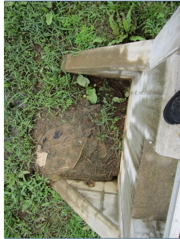
Outlet blockage by sediment
