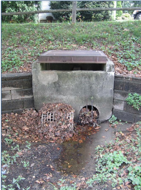
Outlet blockage by debris
