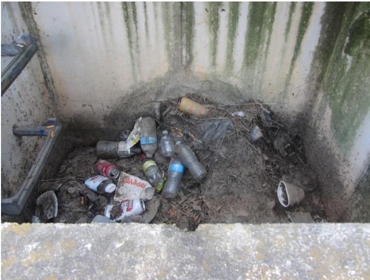
Accumulation of floatables from outfall
