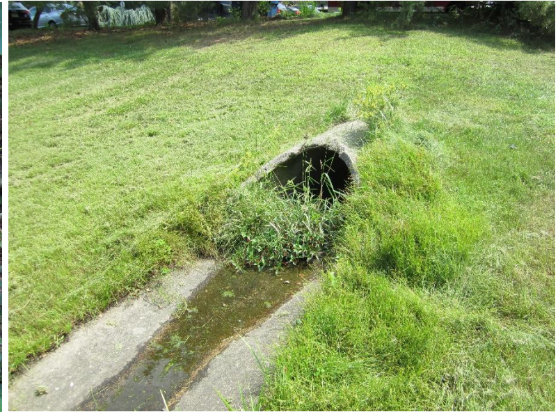
Clogged low-flow channel
